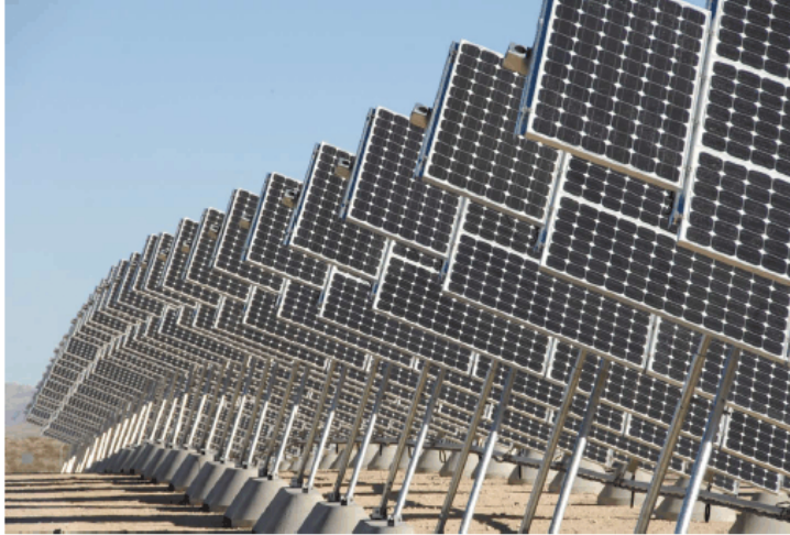
Figure 30. Nellis AFB Photovoltaic Array Detail
